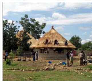
Workers thatch the roof of the first Lubuto Library in Lusaka, Zambia. (Courtesy Lubuto Library Project)
